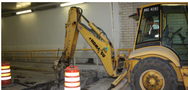
Seaway ARP contractors working on concrete joint repairs in the U.S. Eisenhower Lock Highway Tunnel in Massena, N.Y.
