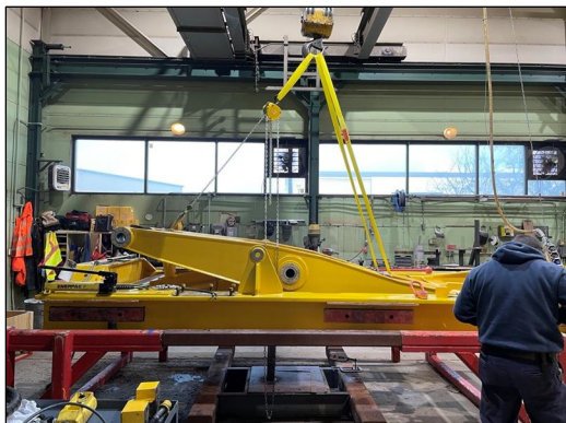
GLS crews perform rehabilitation maintenance on an out-of-service unit of the hands-free mooring system in Massena, N.Y.
