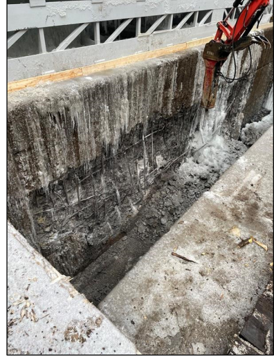
Contractor crews perform concrete rehabilitation work along the stop log sills at Eisenhower Lock to allow additional contractors to complete diffuser replacement work.
