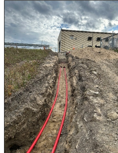
New high voltage power cables located at Snell Lock.
